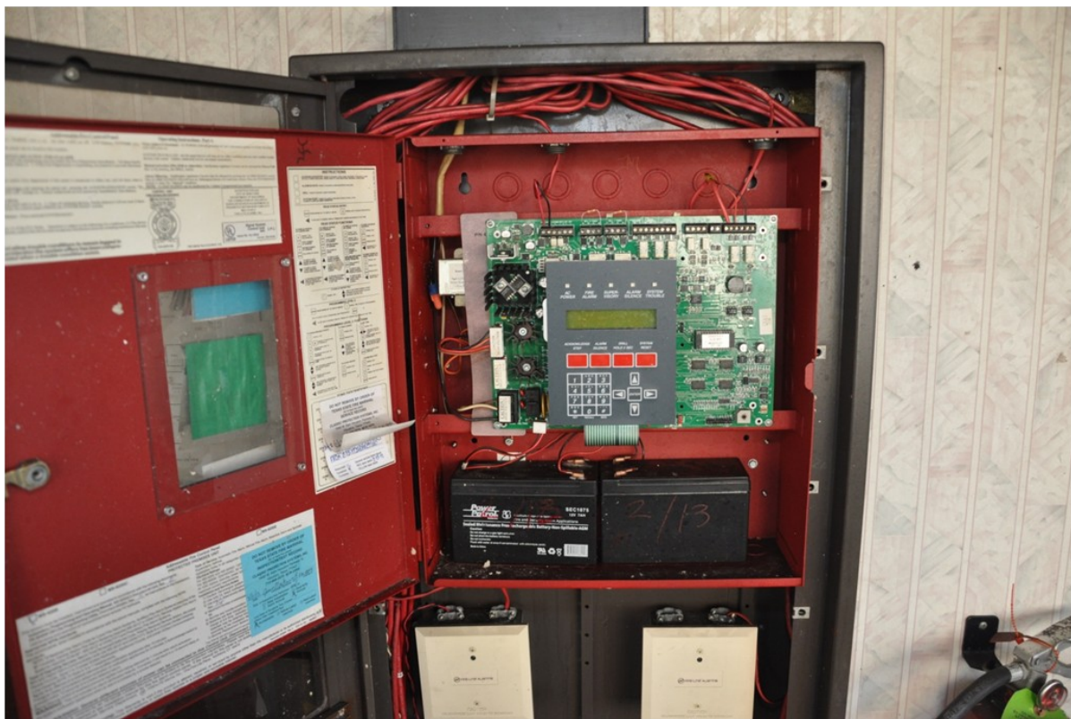
Fire Alarm Panel
