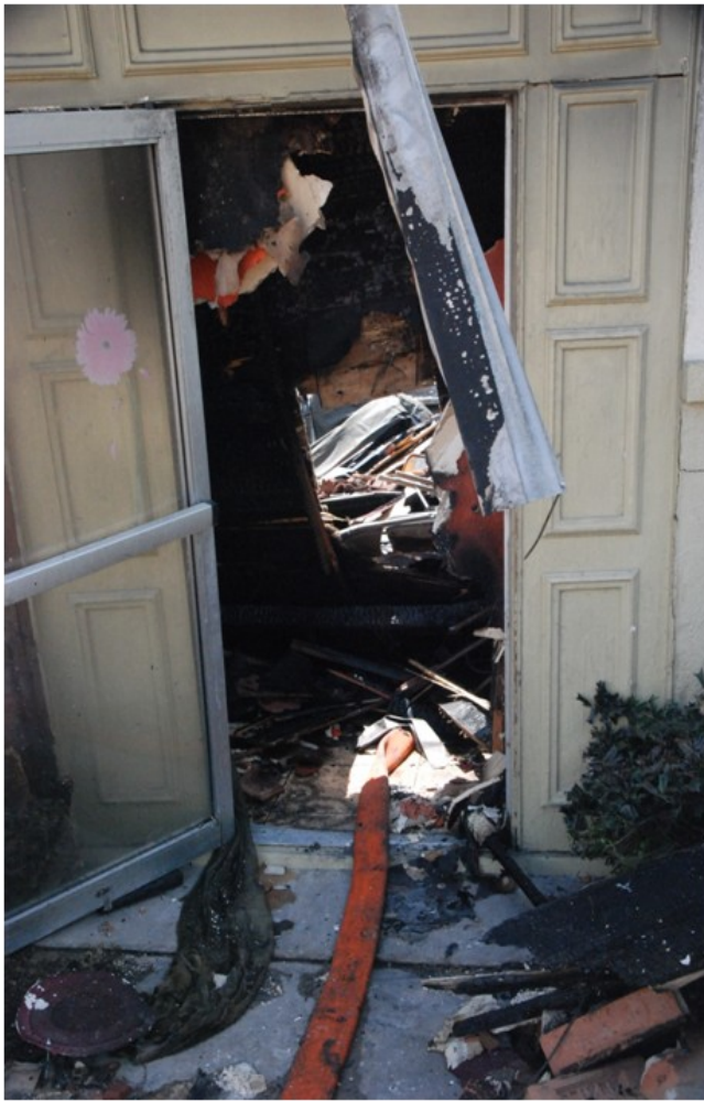
View of the hoseline through the entry door and the hole cut in the roof
