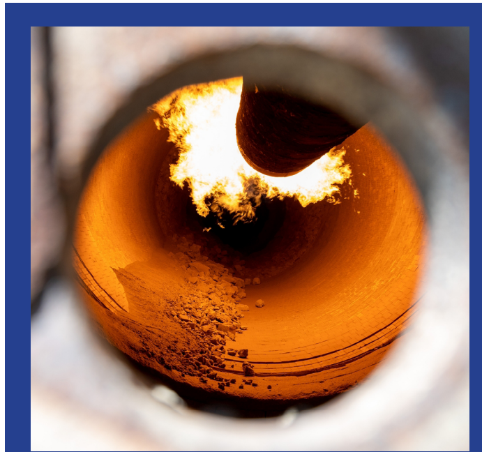
A close-up view through the inspection hole of a rotary kiln used for clinker production in a cement plant.
